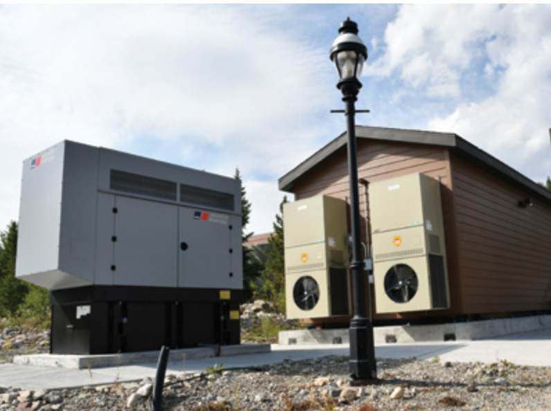
Breckenridge stand-alone Meet-me-Center with air conditioning units and backup power, both requirements for such locations.
